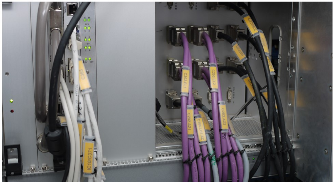
Figure 8: Example of proper identification of cables and sockets/connectors.
