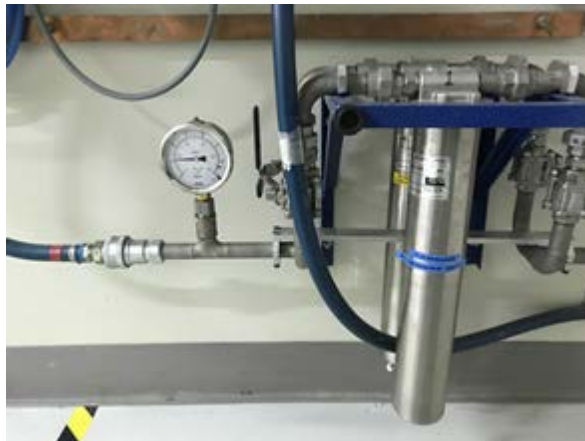
Figure 8: filter pair installed at Paranal
